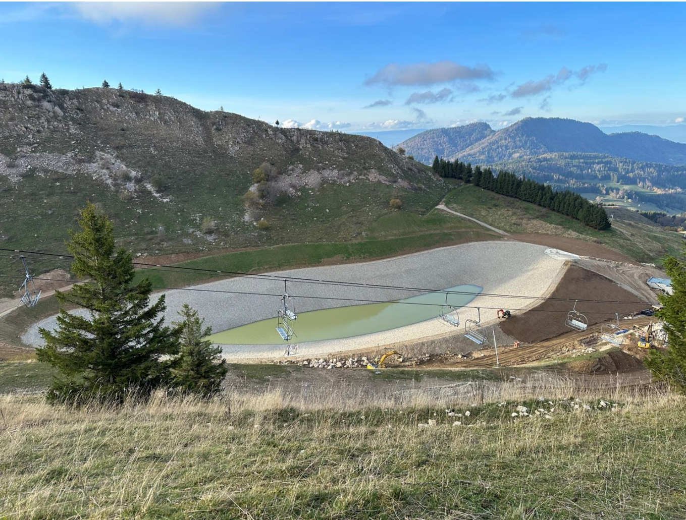
Hill reservoir at the Bellevaux-Hirmentaz station, enlarged in 2022
